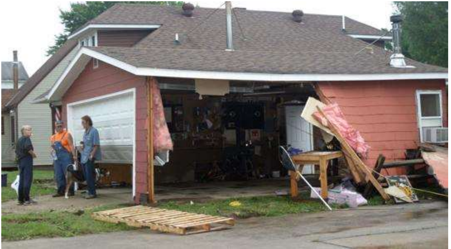
The Bill and LouAnn Wolff house and garage were heavily damaged by floodwaters. Dorothy Robson, Westby Times
