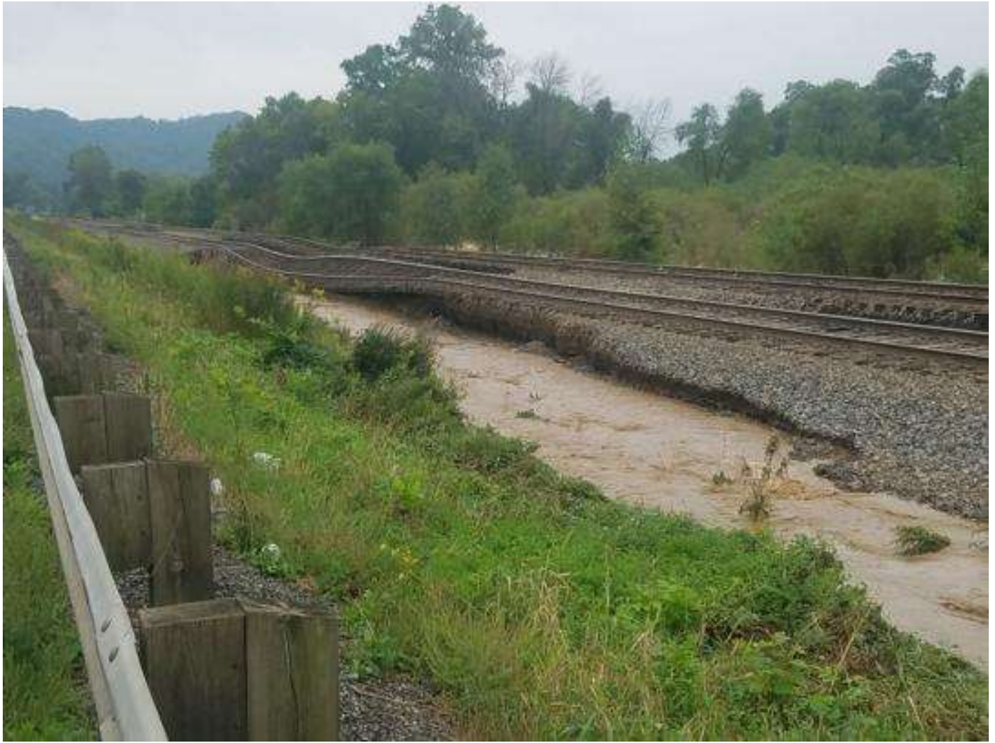
This BNSF rail in the town of Shelby washed out Tuesday morning due to flooding.
