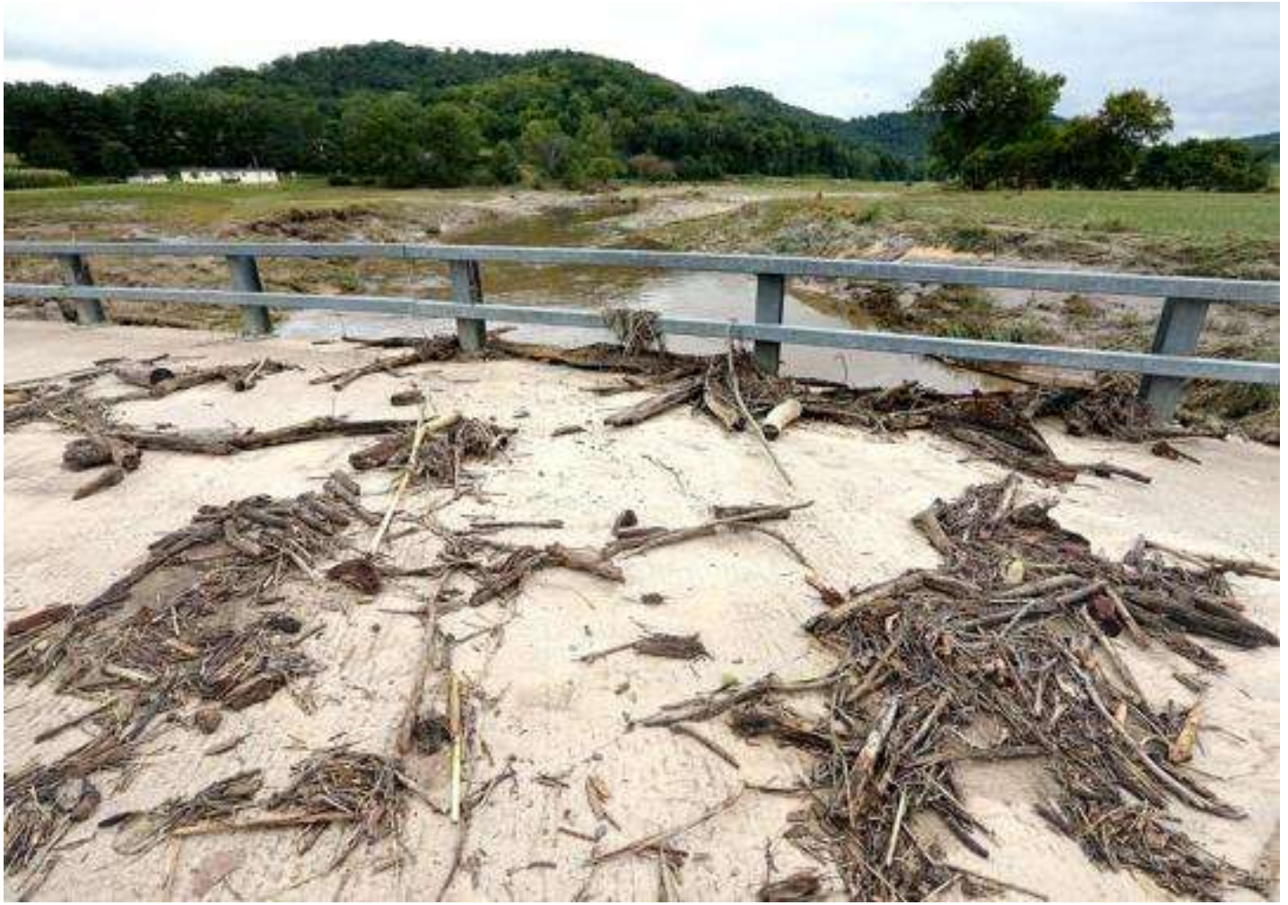
Debris covers a bridge crossing Coon Creek on Knudson Lane in rural Coon Valley Wednesday. Peter Thomson, La Crosse Tribune
