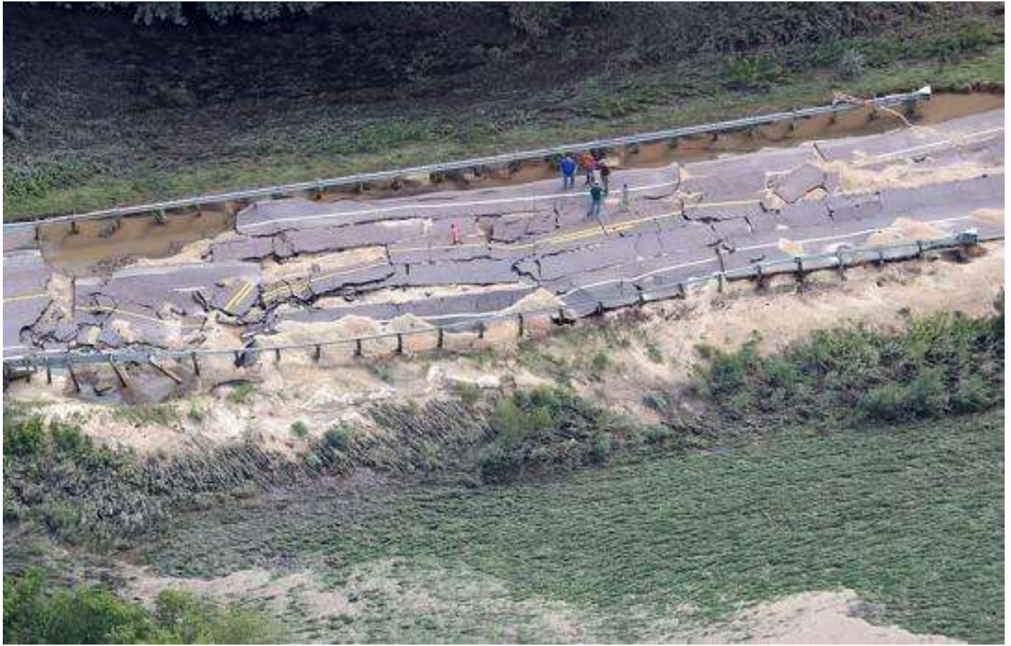
Hwy. 131 near Ontario was one of many area roads to sustain heavy damage in the flooding. Erik Daily
