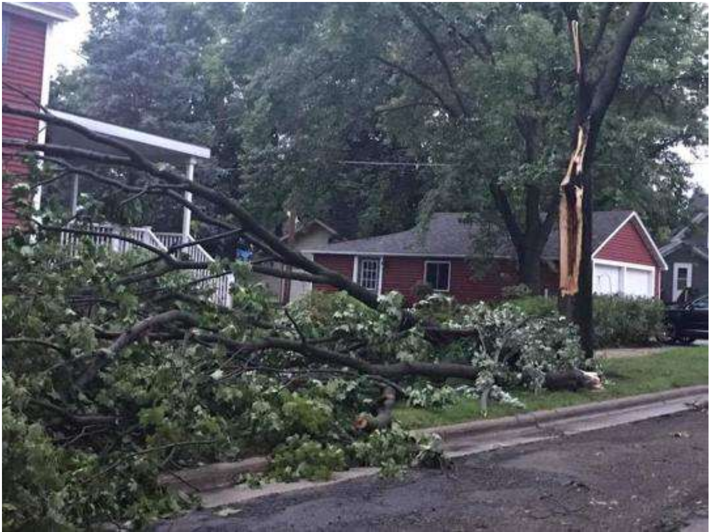
A tree is uprooted in front of a house in Coon Valley.
