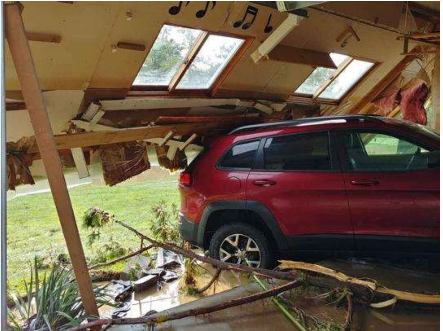
The wall of an attached garage in Coon Valley was knocked out when flooding Monday and Tuesday washed an SUV into it.
