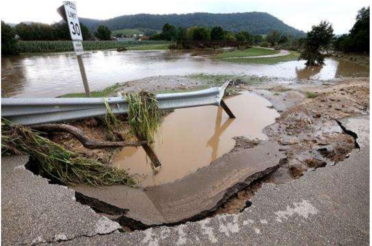
A section of washed-out pavement from Hwy. 14/61 in Coon Valley is seen submerged Tuesday in flood water from Coon Creek.
